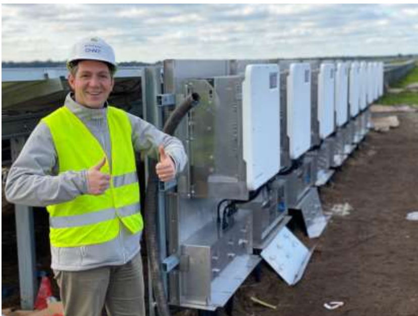
Figuur 45: Head of Engineering & Design controleert de omvormers
